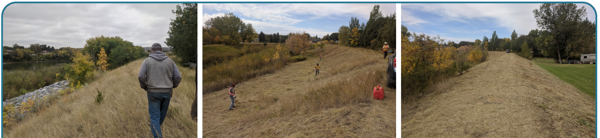
Dike B brush clearing: before (left), during (middle), and after (right), September 2020
