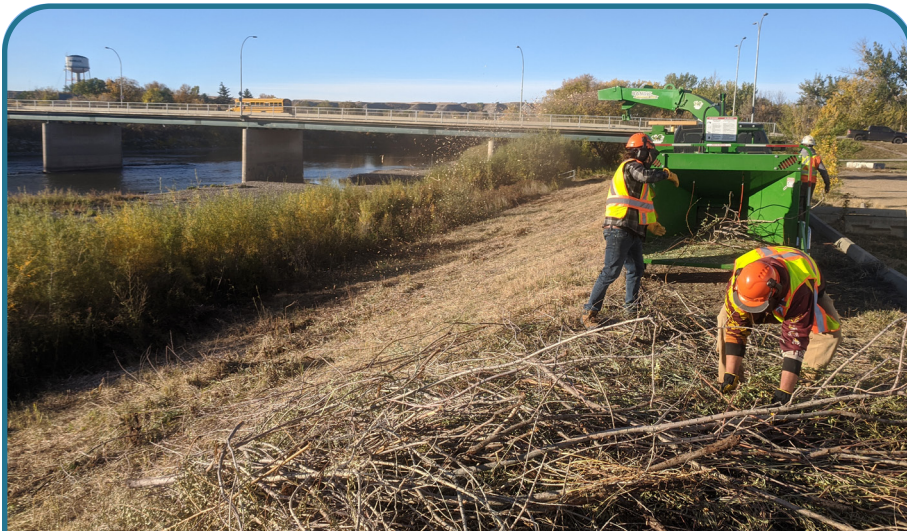
Crews clearing brush and vegetation for provincial dike condition inspection at Dike C, September 2020
