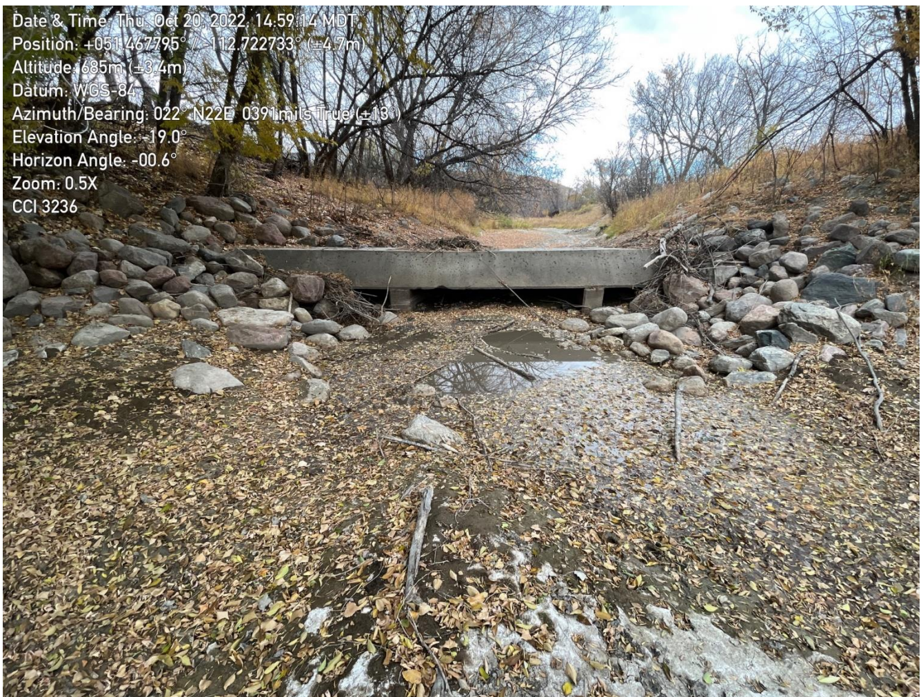
Plate 12. View of sewage feature approximately 340 m upstream of the confluence (October 20, 2022)
