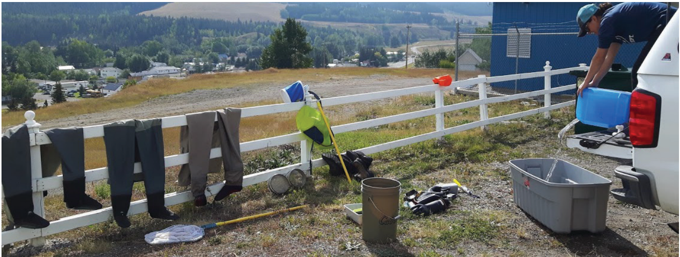
Figure 7: Rinsing and drying field gear using potable water that was brought to the worksite.
